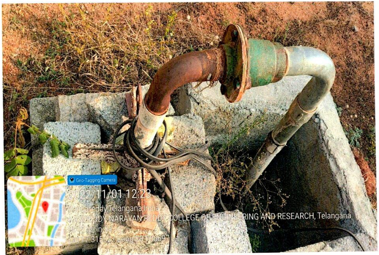
Bore-Well at KNRCER
